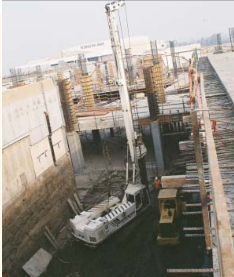
Into this confined area, Magco stuffed our Mait 130 drill rig, Cat 930 loader 75' long tremie and 60 ton Grove Rough Terrain crane.
