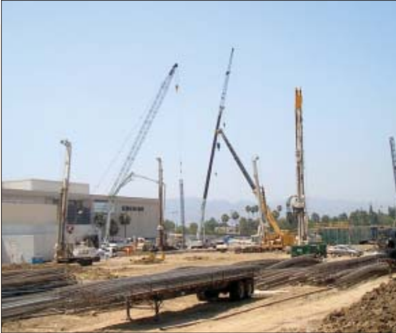
The daily coordination of maintaining production and scheduling material deliveries was challenging.
