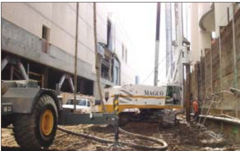
Installing 1,331 Drilled shaft foundations at Westfield Shopping Town Parking Structure Canoga Park, Ca. Magco Drilling's largest drilled shaft project to date.
